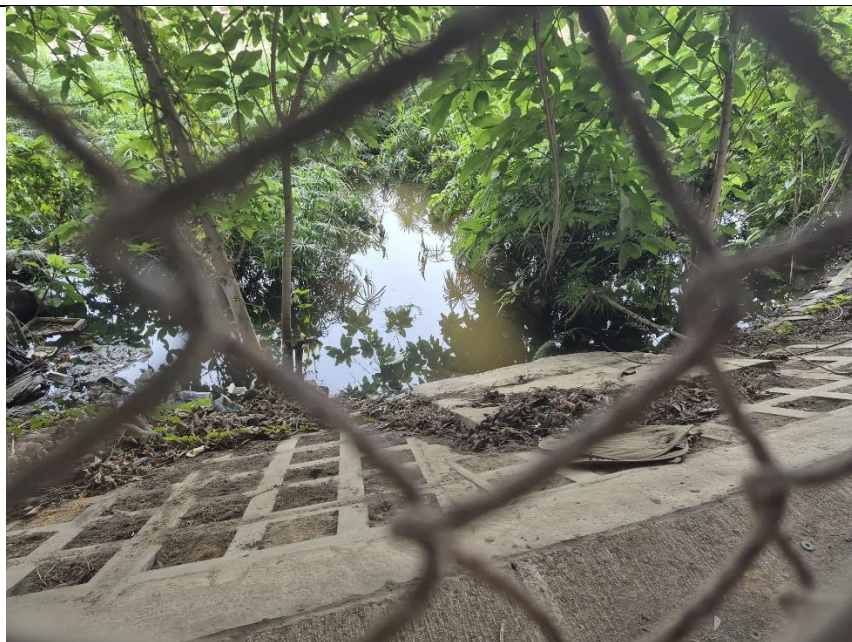
Photo 8 (Taken at Sub Channel under Kong Sham Western Highway near Monitoring station C1 on 12 June 2026)
